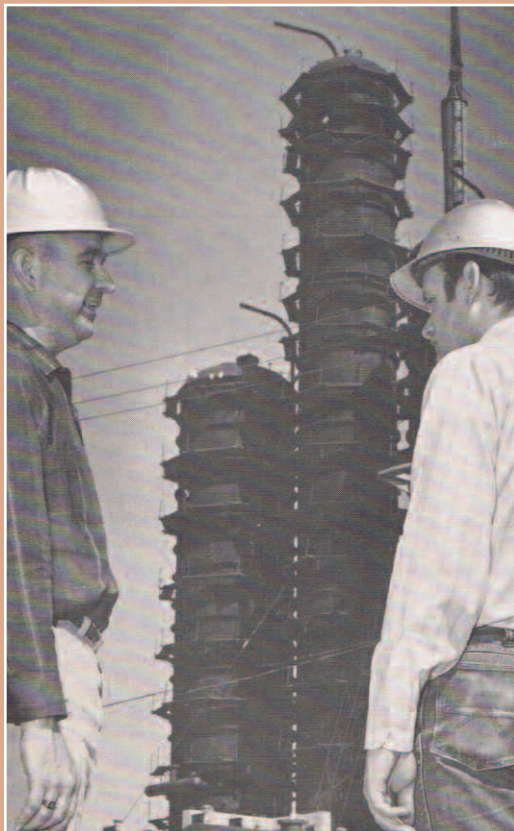
The Chemical Plant's aromatics extraction unit, under construction in the background, was started up in August 1969. In the foreground, operating personnel A.M. Wallingford and Ron Mahaffey discuss construction.
