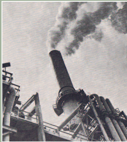
In 1973, a wet gas scrubber was installed on FCCU-2 to improve air emissions from the cat cracker. FCCU-3 would receive its own scrubber two years later.
