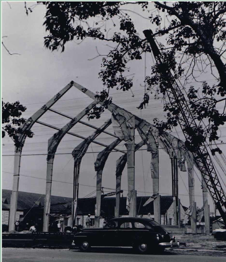
The Refinery continued to help with community activities during the 1950s. Pictured are riggers helping erect beams for Grace Methodist Church.
