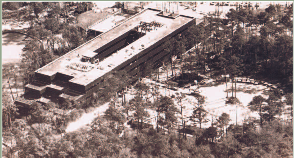
Construction commences on the Chemical Plant Administration Building in 1981. Later known as the Central Administration Building (CAB), this facility would house most of the Complex's management.
