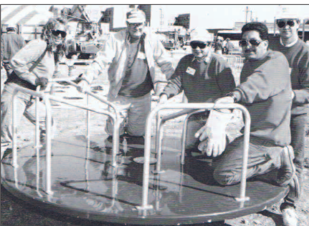
Approximately 150 Exxon volunteers built an extensive handicapped-accessible playground at Goose Creek Park on West Texas Avenue. Pictured are: Camille Borowiak of the Baytown Parks and Recreation Department, Jim Dodson of Basic Chemicals Americas, Reymond Herrin and Robert Villaneuva of the Refinery and Gary Fischer of the Baytown Olefins Plant.
