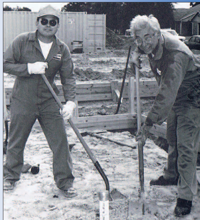
Working on a foundation for Habitat for Humanity are George Cruz, left, and Robert Yznaga.
