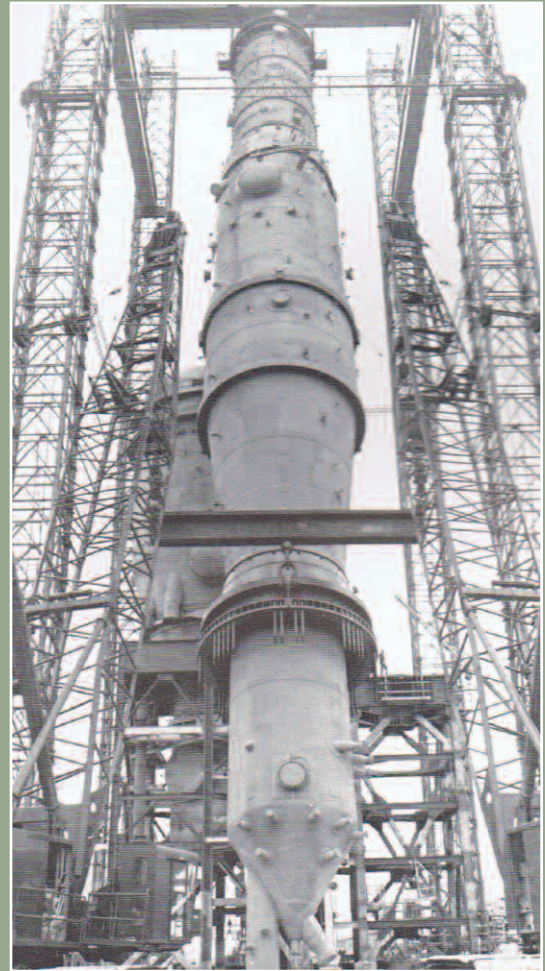
Several vessels that form the core of the flexicoking unit are erected as part of BRUP.
