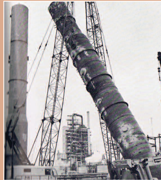
The two main towers at Hydrofiner 3 are raised into place. The unit was officially completed in 1969.
