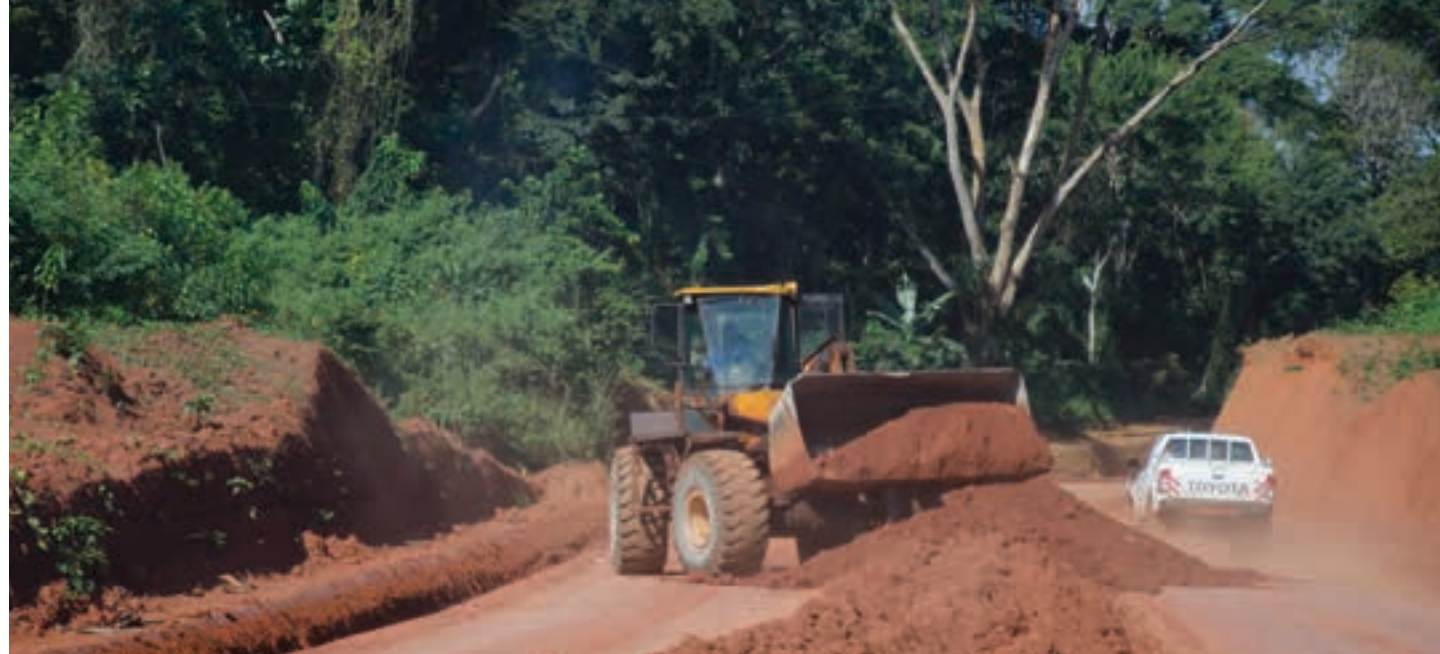
New and improved roads, agricultural activities and other planned infrastructure can all present issues for the pipeline right of way. Careful monitoring of these projects and communication with the government and third parties is key for managing these risks.
