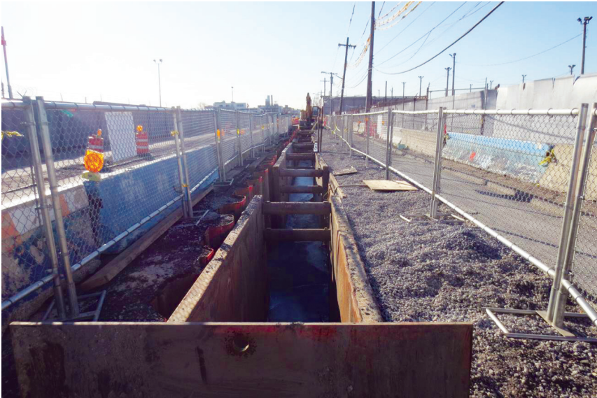
Trenching and bracing completed in preparation for the new storm sewer improvements
