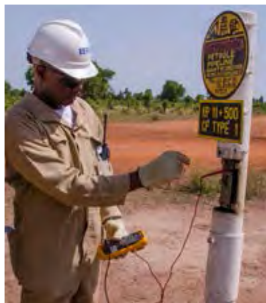
▲ Close interval monitoring of the cathodic protection system can be used in conjunction with inline inspections to protect against corrosion - all while oil continues to flow.
