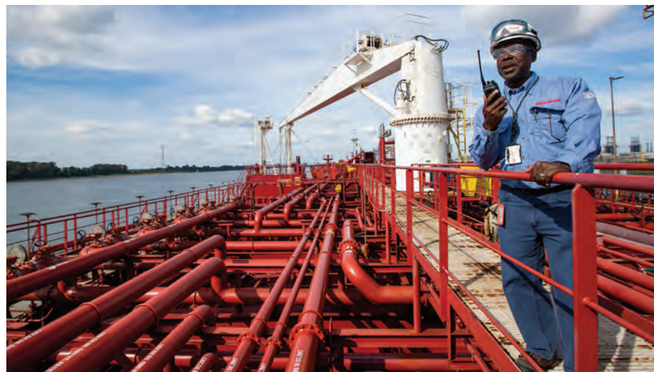
Derrek Lathon, marine dock supervisor, communicating equipment observations with his team at the ExxonMobil Baton Rouge refinery.
